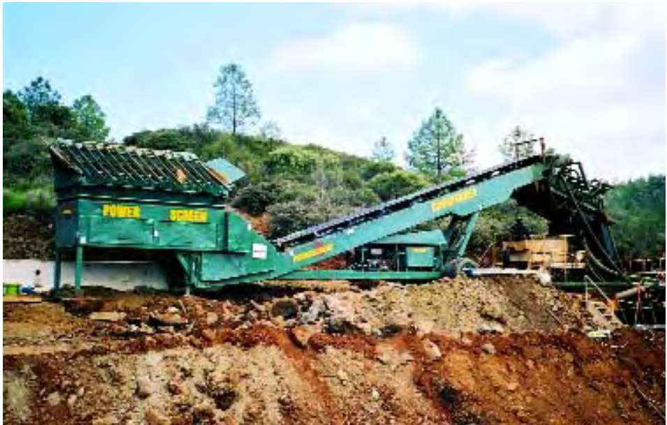
Figure 7. This new processing plant was installed at the Benitoite Gem mine in spring 2002. Material is dumped into the hopper (far left) and proceeds up the conveyor belt to a washing/screening apparatus (top right). Mineral specimens larger than \frac{3}{4} inch (1.9 cm) are hand picked from the conveyor belt on the far right. Smaller material is sent through a jig system, which is partially visible (tan-colored box) below the screening apparatus. Benitoite concentrate, down to 2 mm, is removed from the jigs each day. Photo by Bryan Lees.
